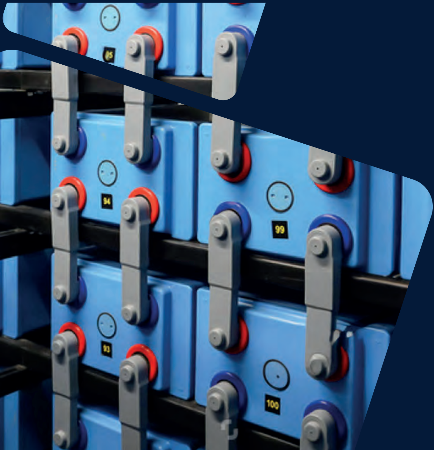
Ups & Battery Rooms
